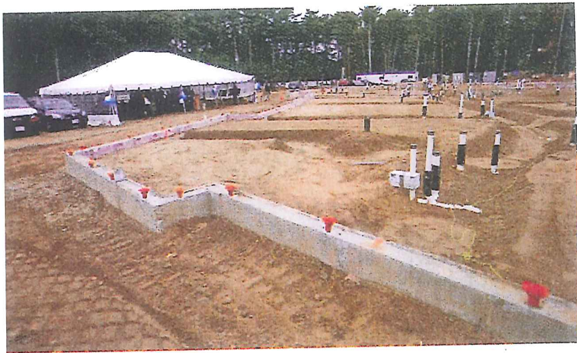
EG DERR/ The Patriot Ledger Concrete foundations are in place for Barstow Village in Hanover, an affordable housing complex for seniors expected to open early next year.
